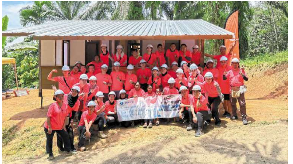
Zurich Malaysia in collaboration with EPIC Homes, embarked on their first house-building project of the year at Kampung Orang Asli Bukit Manchung, Bukit Beruntung.
