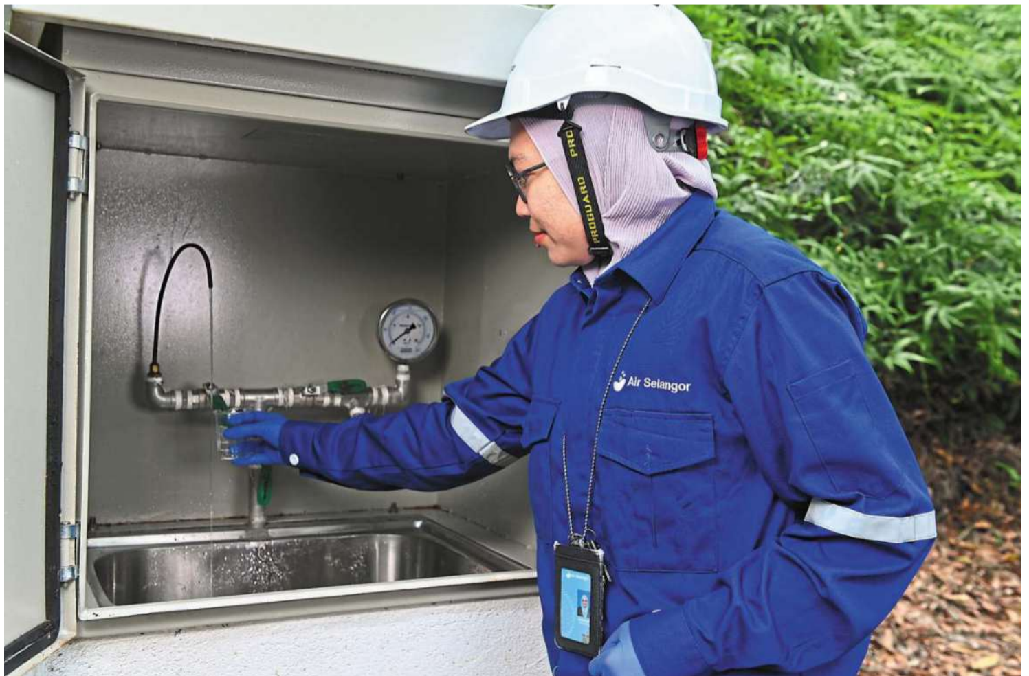
Air Selangor conducts regular water sampling and analysis at its treatment plants, with samples tested every two hours by a team of chemists and microbiologists to identify and address any impurities or contaminants before the water is distributed to the public.
